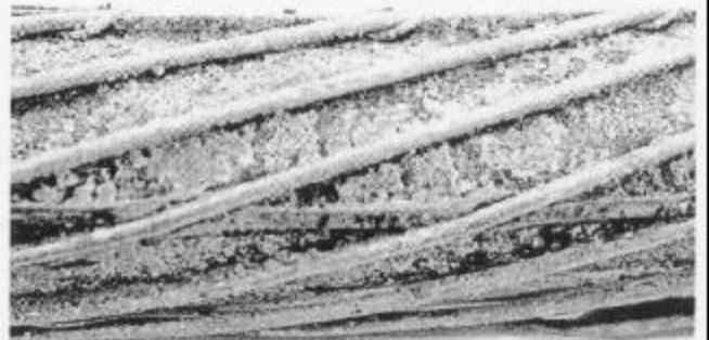
Figure 5. Unjacketed power distribution cable with outer shield wires encrusted with dried soil, causing the space between the shield wires and the semiconductor outer layer of the cable to have high resistance. Reproduced with permission from figure 8 of paper by S. Boggs (ref. 14).
